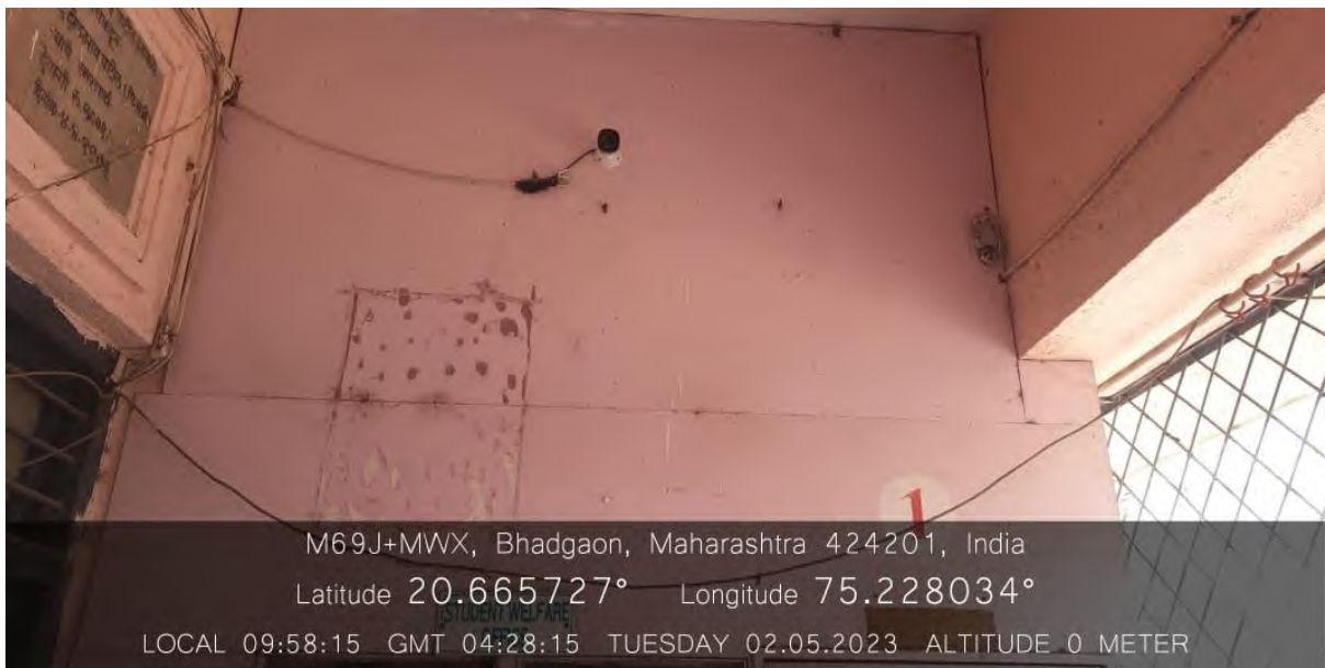
CCTV Camera in Old Campus
