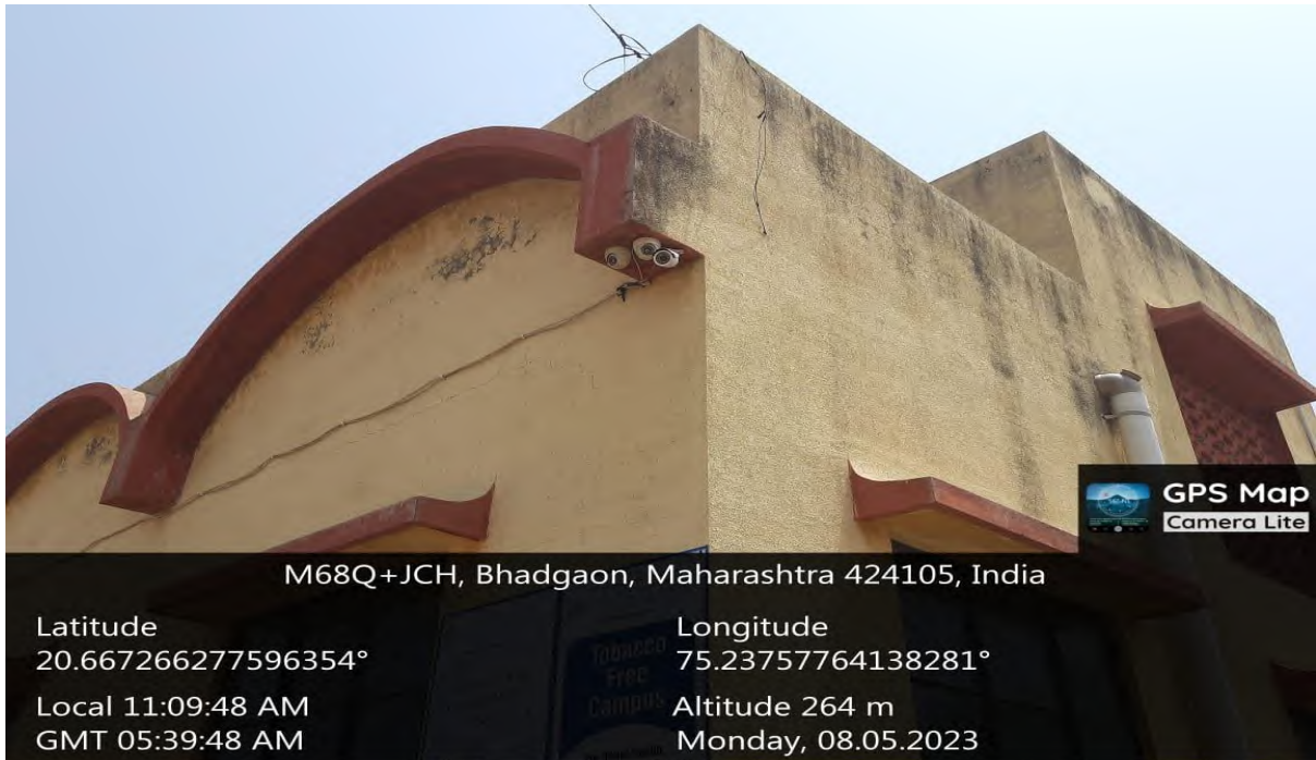
CCTV Camera in New Campus
