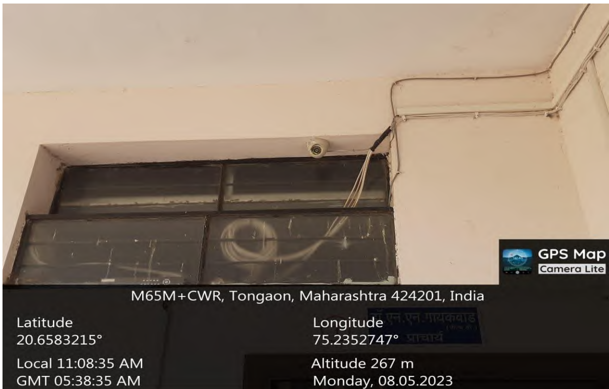
CCTV Camera in New Campus
