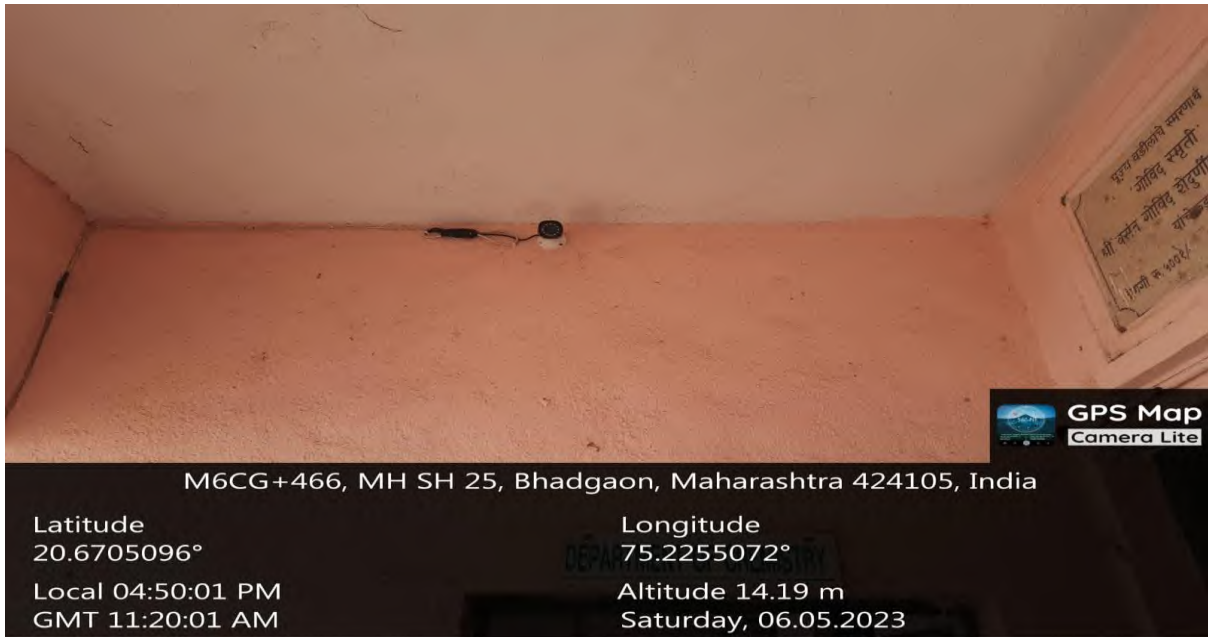
CCTV Camera in Old Campus
