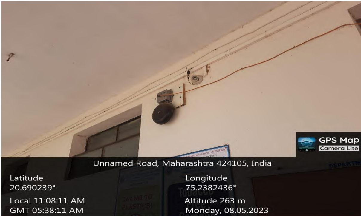
CCTV Camera in New Campus
